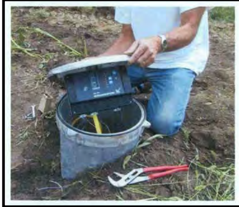
Controls mounted on plate attached to lid
